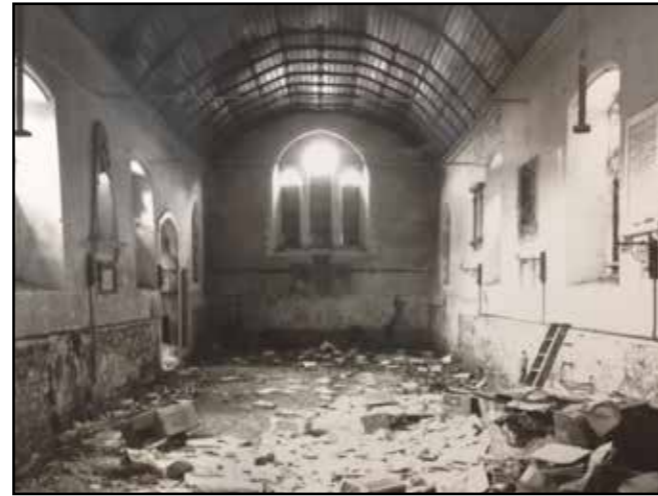
St Andrew’s showing bomb damage. The photographer is not known
