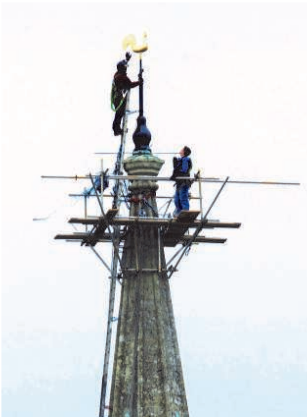
Adrian Tarrant and his team restoring the weathercock to its original position
